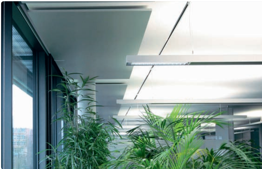
VARICOOL velum as edge strip elements in combination with CCTC (installation next to the façade).
